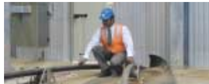
Project Director Mike Farr with cables as they enter the Berri Converter station after 176 km underground
