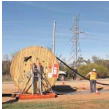
The old and the new ... Murraylink underground cable rollout (foreground), with older style overhead cable lines behind
